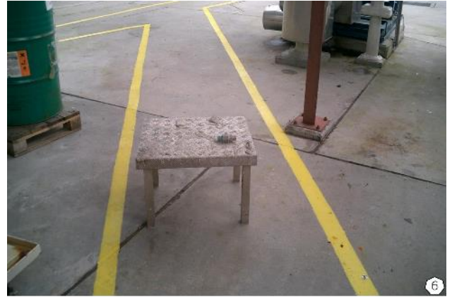
6) Equipment located in an escape route may allow the incident to escalate further.
