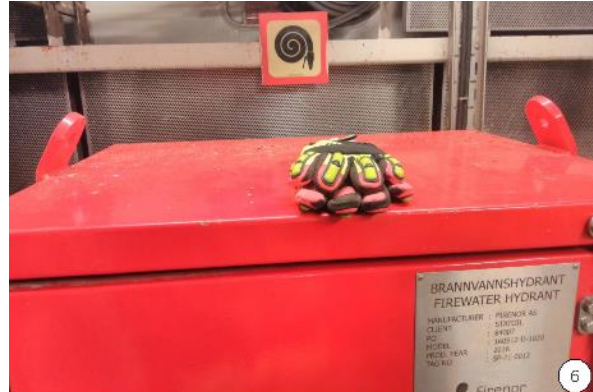
6-Gloves left behind in a room with pump systems; these may block the pump system in the event of a massive influx of water
