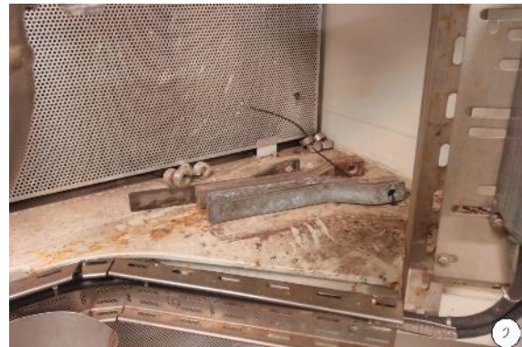
2-Loose metal objects in room with watertight doors. In a worst case scenario these may become trapped between the door and the frame.
