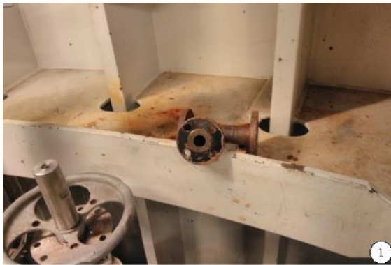
1-Loose flange may fall onto the float. This may prevent the water alarm from being triggered.
