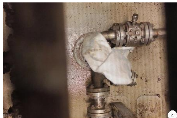
4-Cloth below the flooring in a room with pump systems
