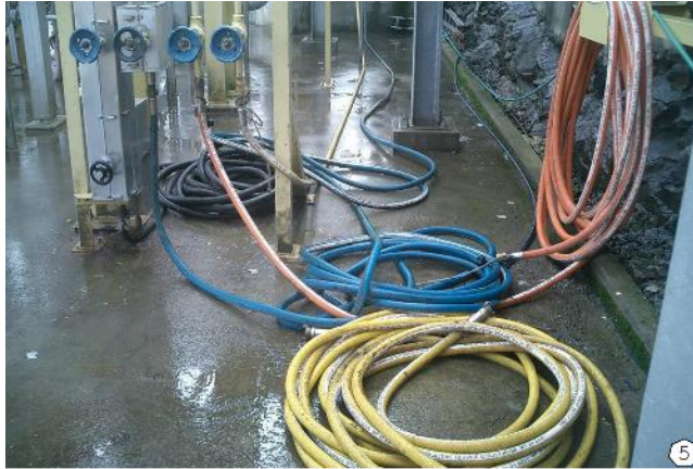
5) Hoses will prevent access in an emergency situation. May allow the incident to escalate further.
