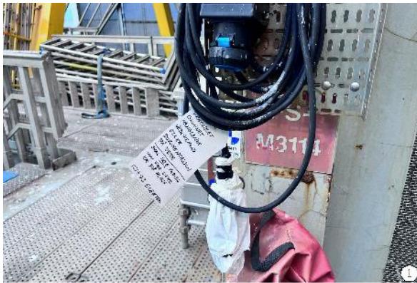
1-Fire and gas panel utkoblet.
